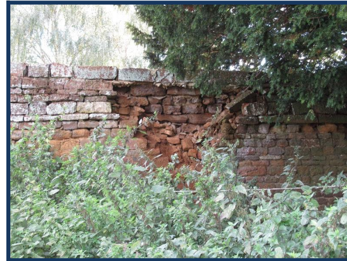
Figure 44: Damage to 16 th century wall
